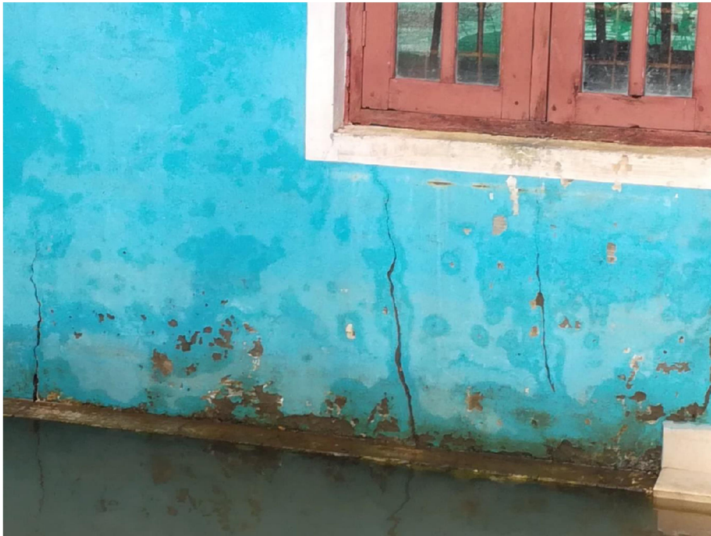
Figure 2 Structural Damage Analysis of Houses
