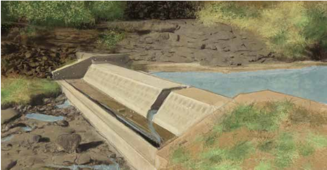
Figure 8.14: A cement check dam across a ephemeral stream to store water in semi-arid region
